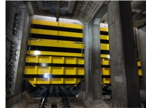
Flood prevention gate at tunnel outlet
