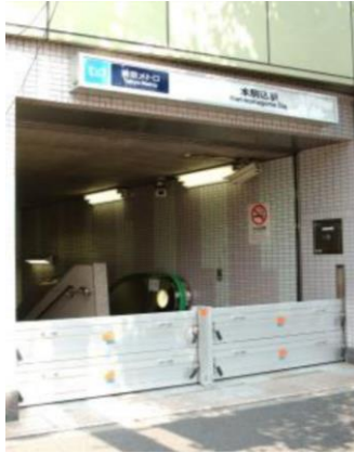
Flood prevention stop boards
